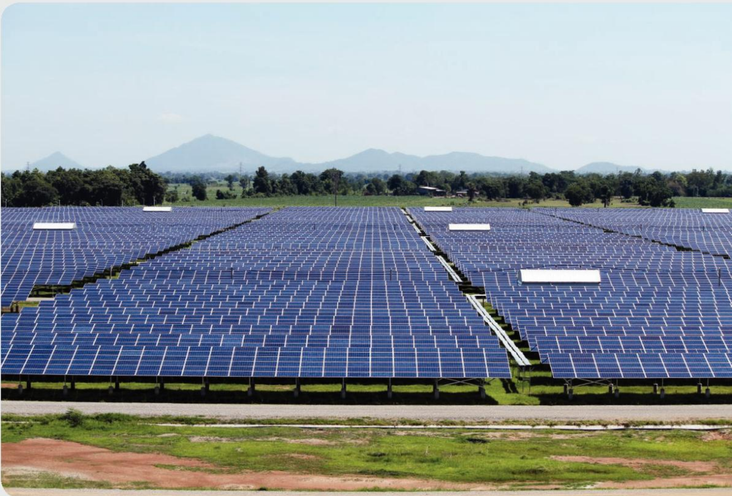
▲ A solar farm
